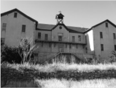
The threats to historic buildings on the former St. Catherine's Indian school campus have received OSFA's attention and action for several years now..
